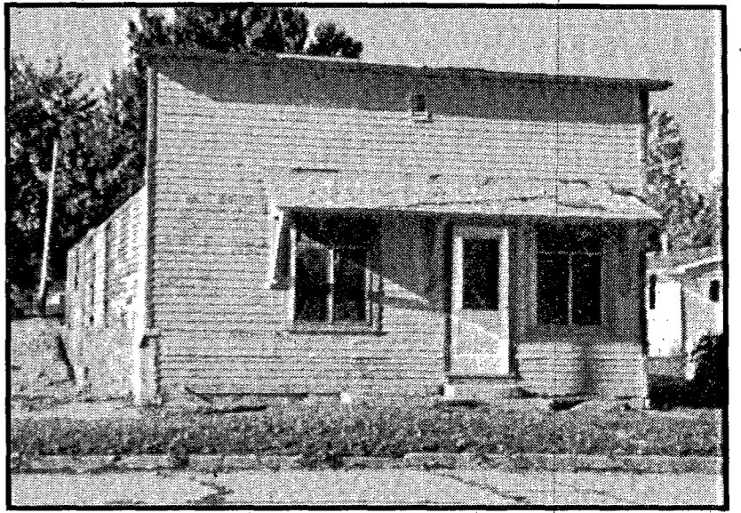
Proceeds from the fundraiser will help repair this building for displaying medical equipment and home furnishings.
