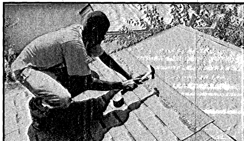
Buay Gatluak, a Wayne State College student, worked on the roof of the Habitat for Humanity house this past Saturday.
